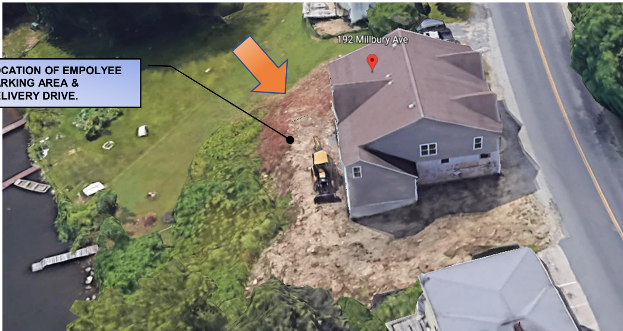
ORTHO PHOTO 02: Project Fill Area for Parking and Storm Drainage Detention System, VIEWING NORTHWEASTERLY (GOOGLE EARTH2019)
